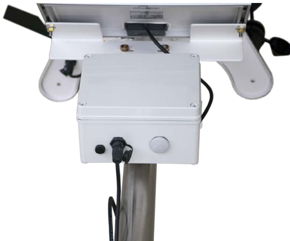
FIGURE 5-21. 18971 cable connected to auxiliary battery enclosure
