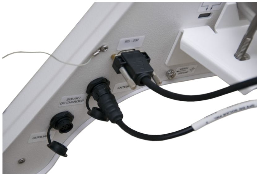
FIGURE 5-18. Short haul modem cables connected to TurfWeather station
