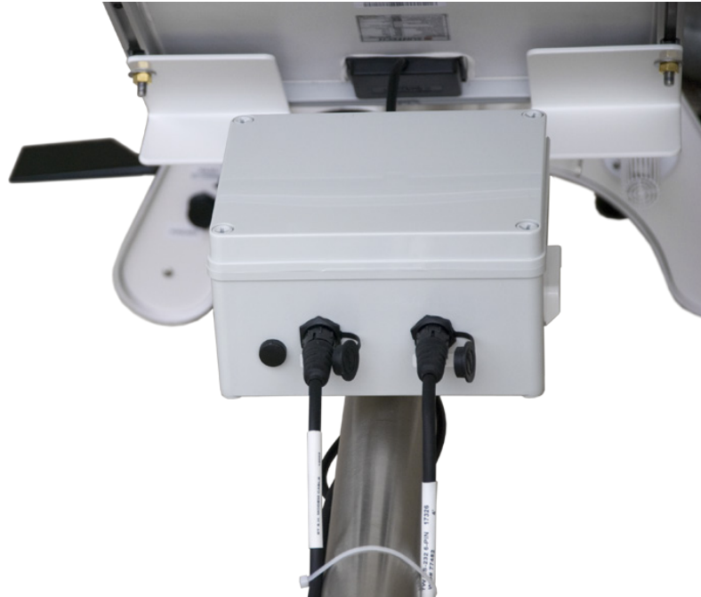
FIGURE 5-17. Cables connected to enclosure for short haul modem
