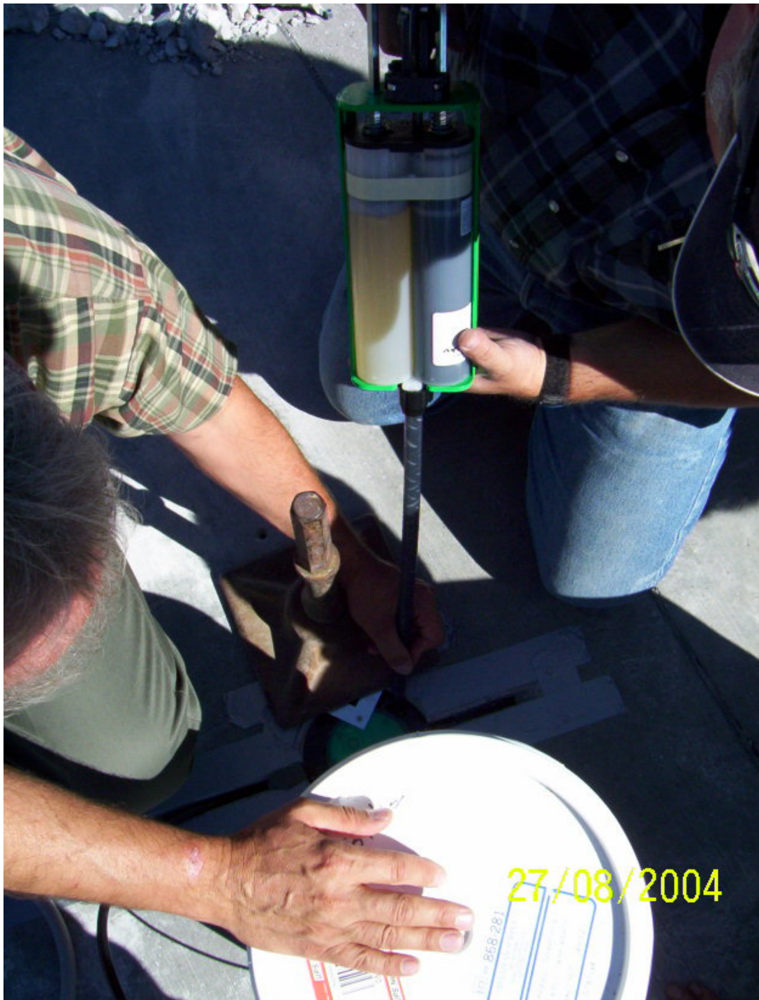
FIGURE 3-6. First pour of Fabick epoxy, pn FJS (fast set), useable between 20° to 180°F.
