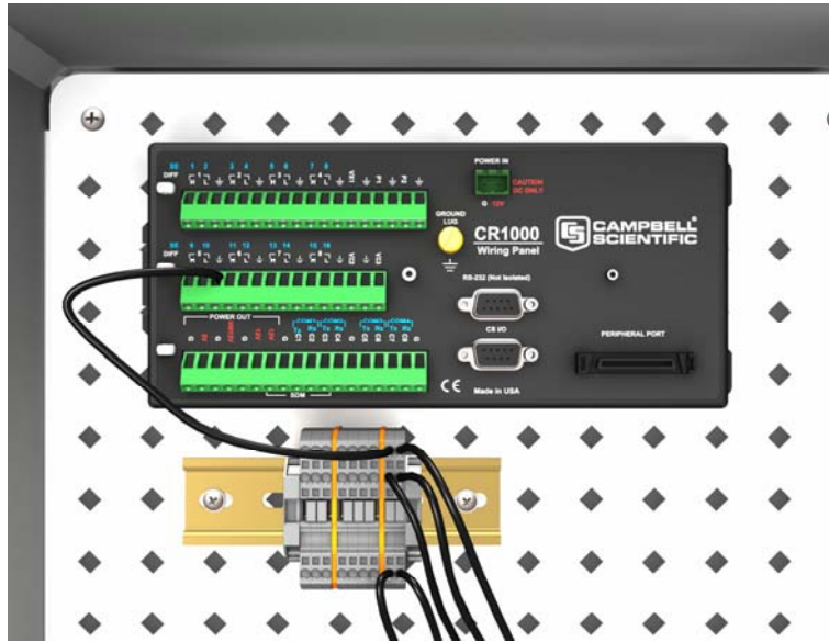
FIGURE 6. An Installed and Wired 25458 DIN Rail Terminal Kit
