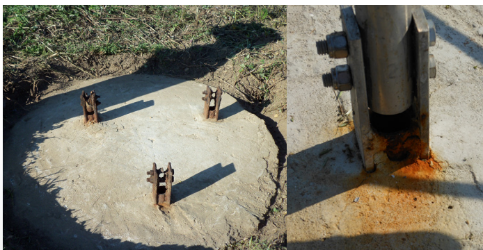
Figure 2: Corrosion in a coastal environment
