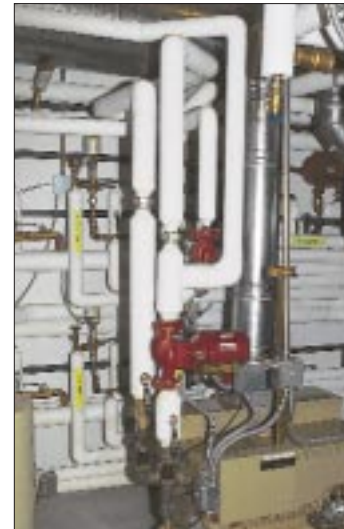
Systems can monitor and control pumps, fans, and starter motors. Proportional control of dampers is also possible.
