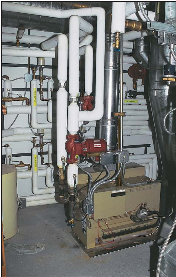
The CR23X monitors and controls the pumps, fans, and starter motors in an HVAC system.
