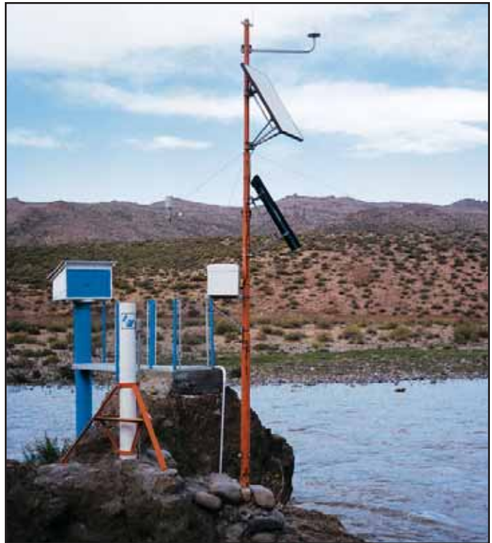
A satellite transmitter provides telecommunications for remote Argentine stations where phone lines are impractical.
