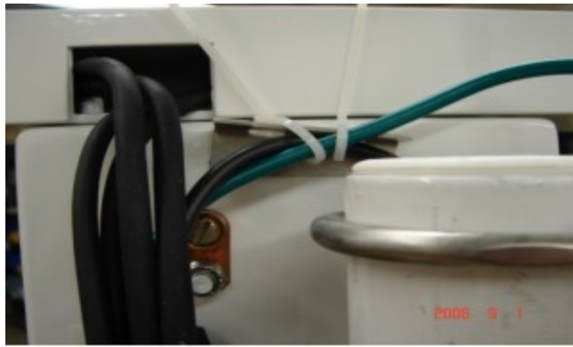
FIGURE 6-28. Loosely wire tie antenna cable
