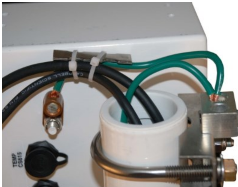
FIGURE 6-39. Grounding to lightning rod clamp
