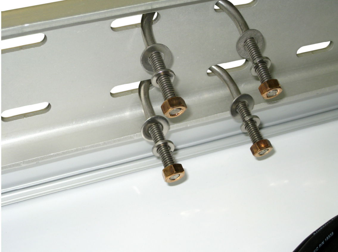
FIGURE 10. Lock Washers and Flat Washers are Used to Secure the Two 5/16-18 x 2.0 U-Bolts to the Solar Panel Mount
