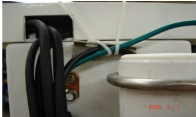
FIGURE 6-28. Loosely wire tie antenna cable
