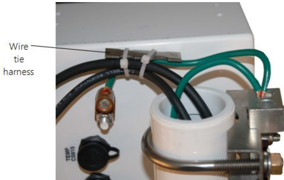
FIGURE 6-46. Cabling strapped to wire tie harness
