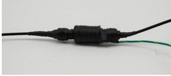
FIGURE 8-14. Properly Weather-proofed Antenna Cable Connection with Surge Protection
