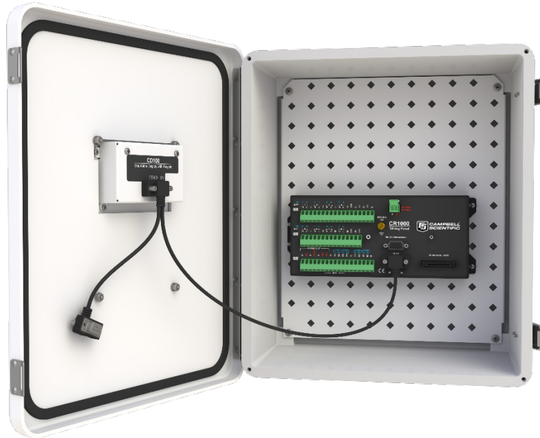
FIGURE 3-1. Connecting the CD100 to the CR1000 datalogger
