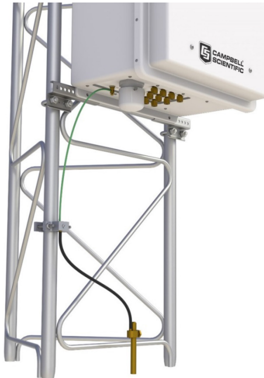
FIGURE 5-10. AP200 earth grounded on a UT30 tower
