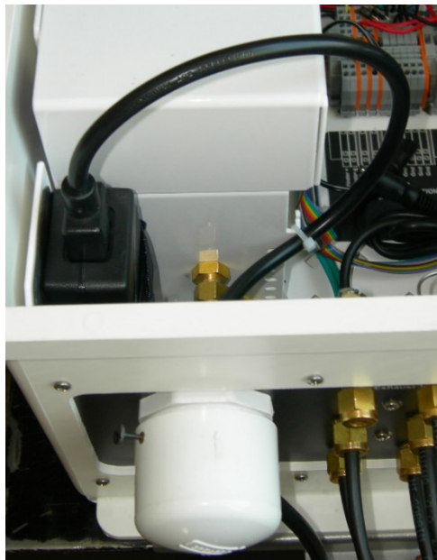
FIGURE G-4. AC power cord secured within AP200 system enclosure
