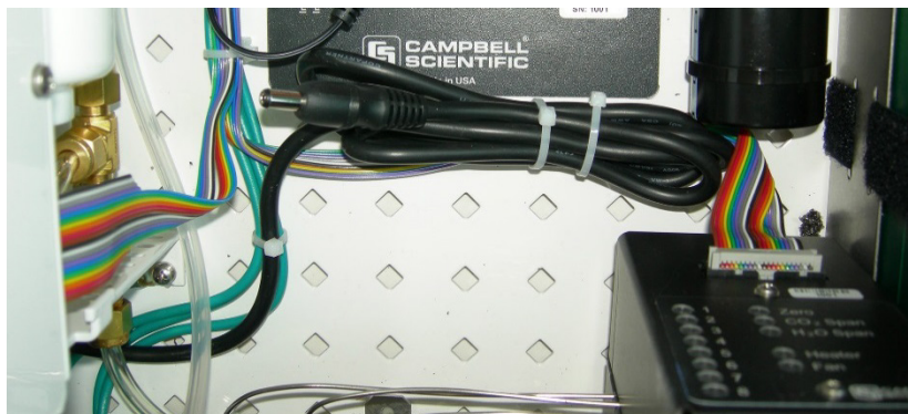
FIGURE G-2. Bundled cable of power adapter
