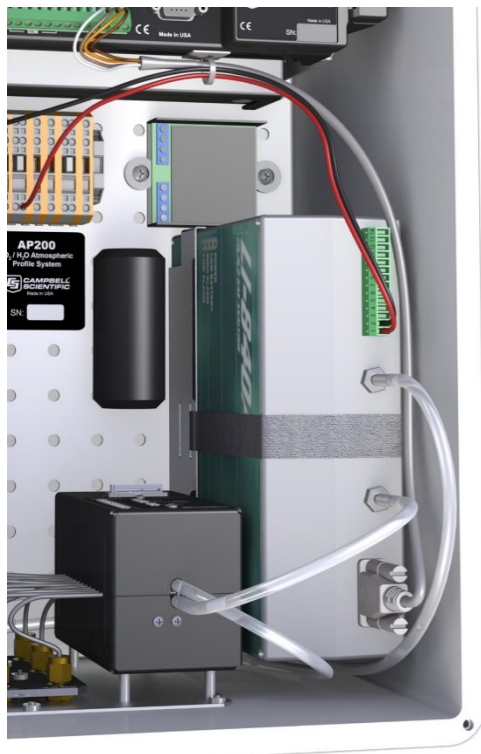
FIGURE 7-4. Installed IRGA in system enclosure
