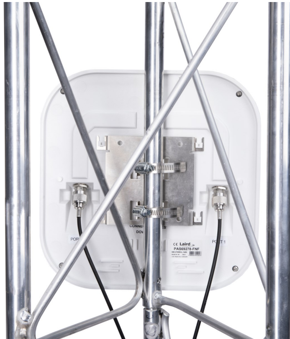
FIGURE 5-2. 38485 mounted on a tower
