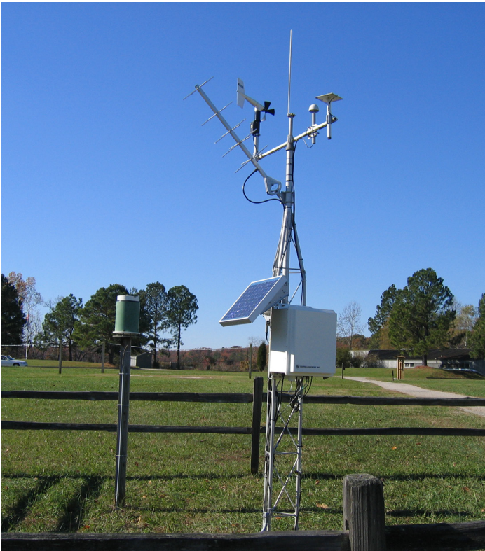
This station for the National Estuarine Research Reserve (NERR) in Virginia transmits data using a satellite transmitter.
