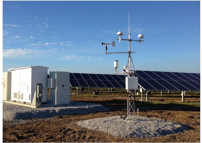
An automated weather station for solar-farm performance monitoring. This turn-key system was customized by Campbell Scientific to meet the specific requirements for Ontario solar farms.
