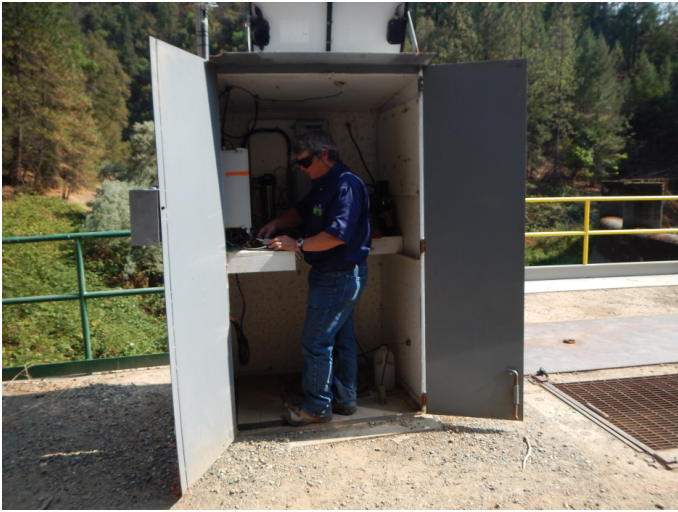
Michael McCool of GWS installing CR800 in instrument shelter (Photo courtesy of Ryan Coursey-Willis)
