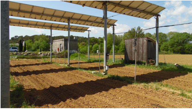
Monitoring of radiation, rainfall, air temperature, and humidity under photovoltaic panels (CR1000 datalogger, SP1110 radiation sensor, CS215 thermo-hygrometer, 52203 rain gauge)
