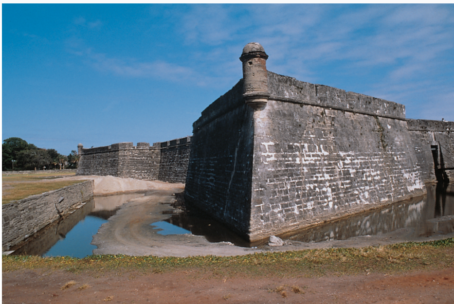
Castillo de San Marcos National Monument, St. Augustine, Florida. Taken in 1995, this view looks across the moat toward the southwest bastion, where several major cracks are visible.
