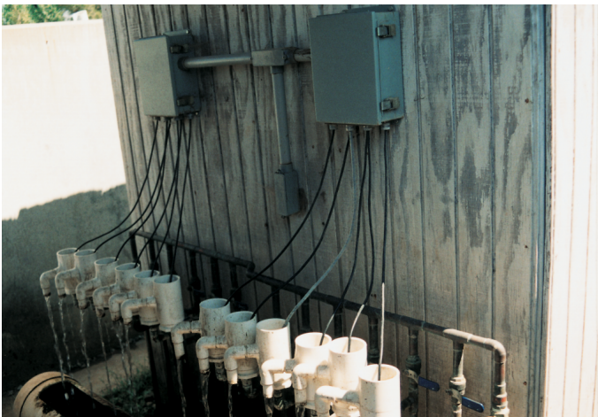
Rather than deal with the added expense of extra cable lengths for 12 individual dissolved oxygen probes, Stolt Sea Farm devised a system in which water continuously flows from the tanks through PVC pipe to sensors at the monitoring station.
